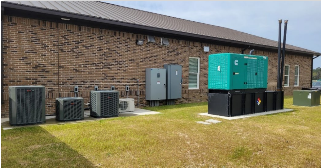
Figure 6. Existing Electrical & Mechanical Infrastructure
